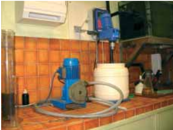
PMA Series used for sampling in the control process at a waste water treatment plant
